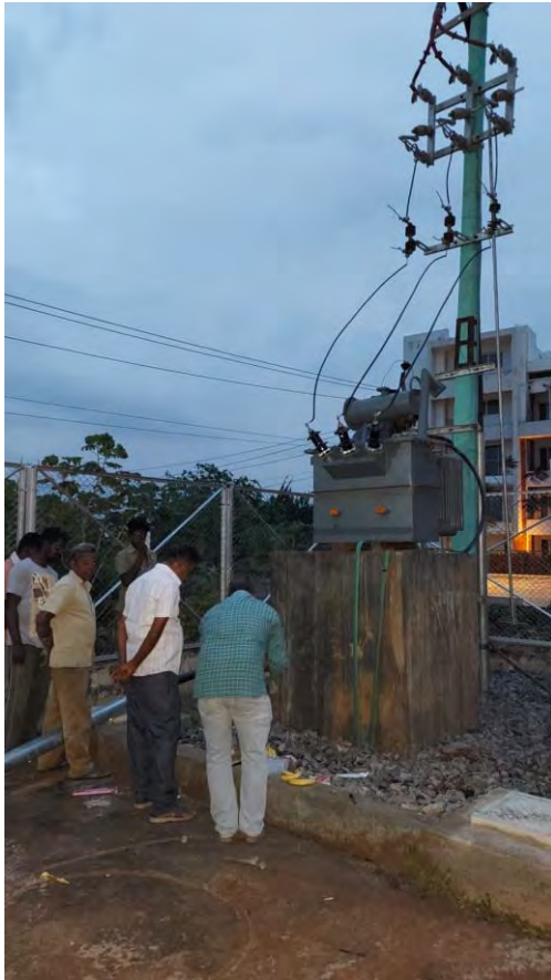
TC YARD-1 TRANSFORMER POWER CHARGED
