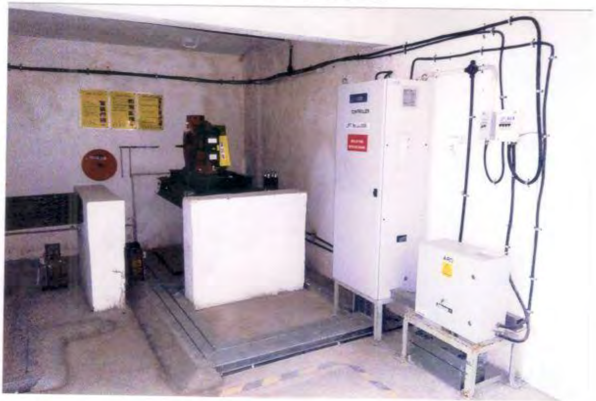
Lift Machine Room
