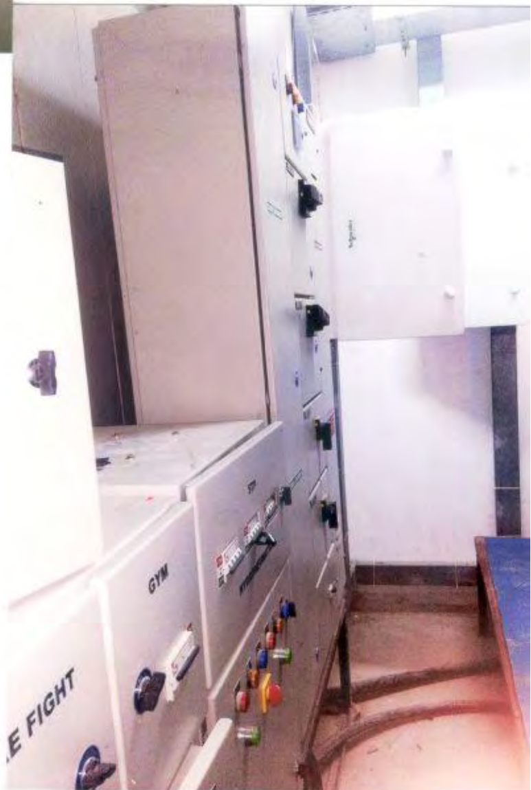
Fire Fighting Pannel →
