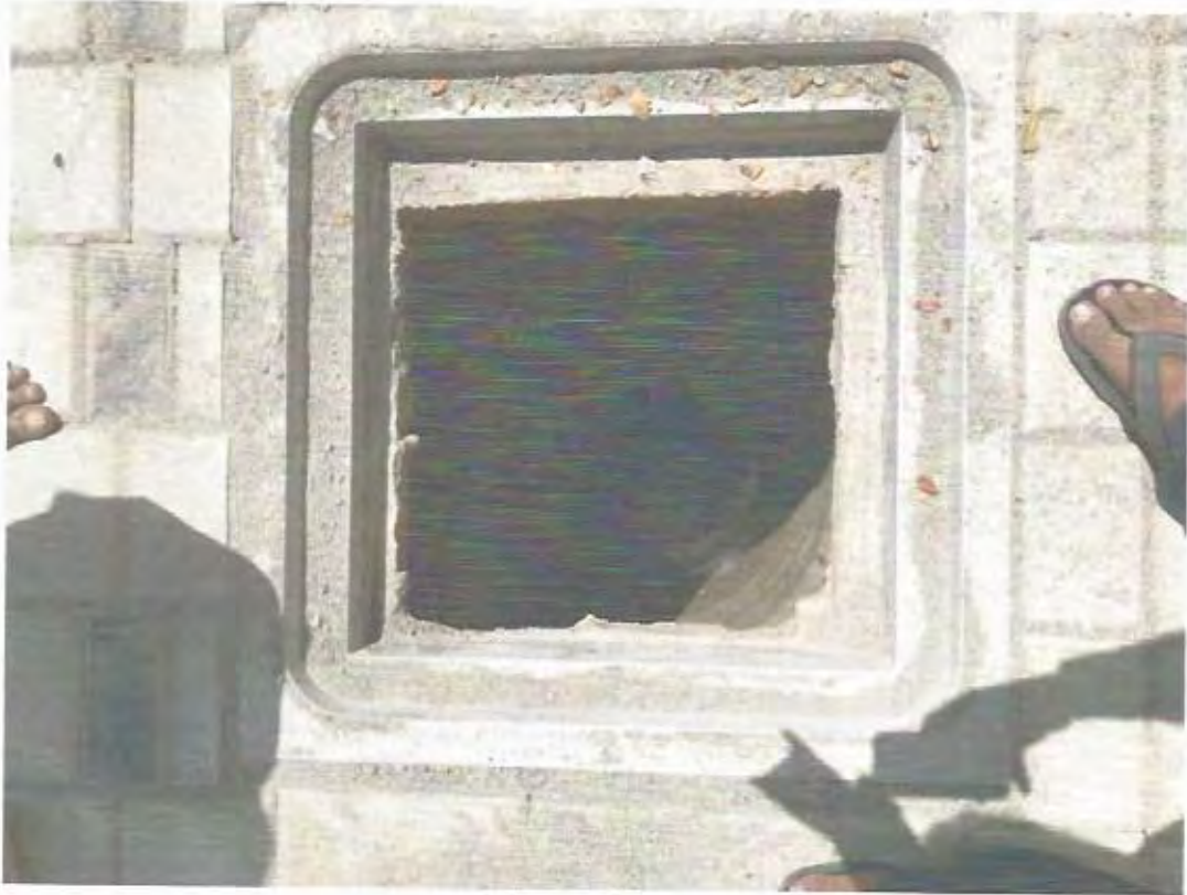
Rain water harvesting open & closed photos
