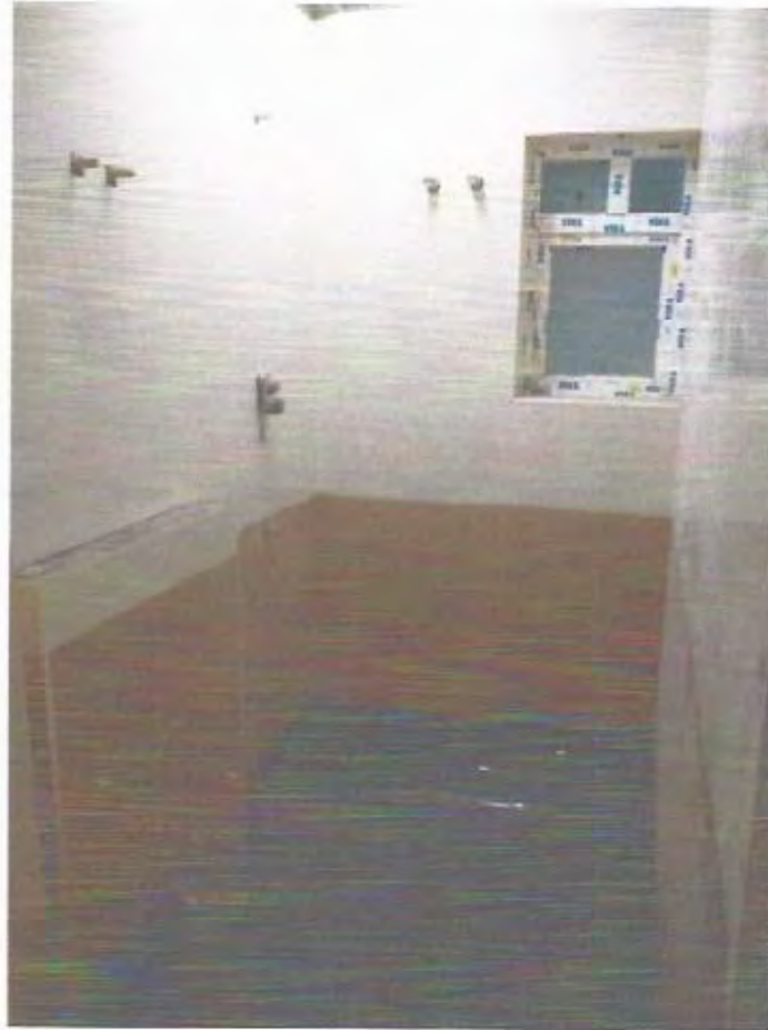
Bathroom including ventilator
