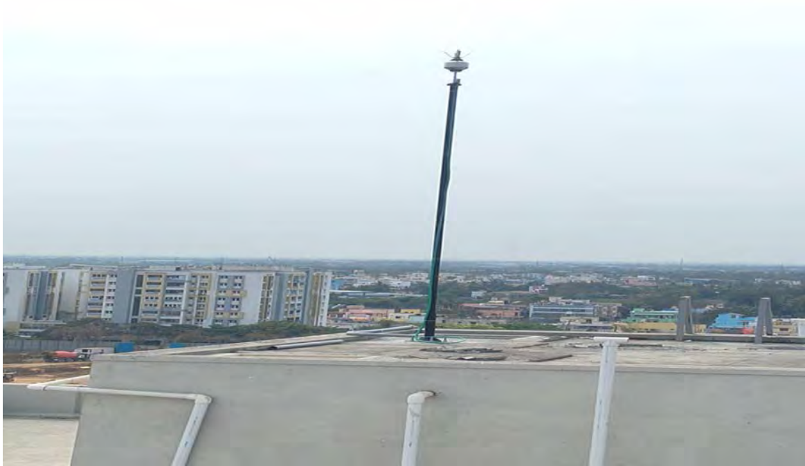
Lightening arrester in D1 Block
