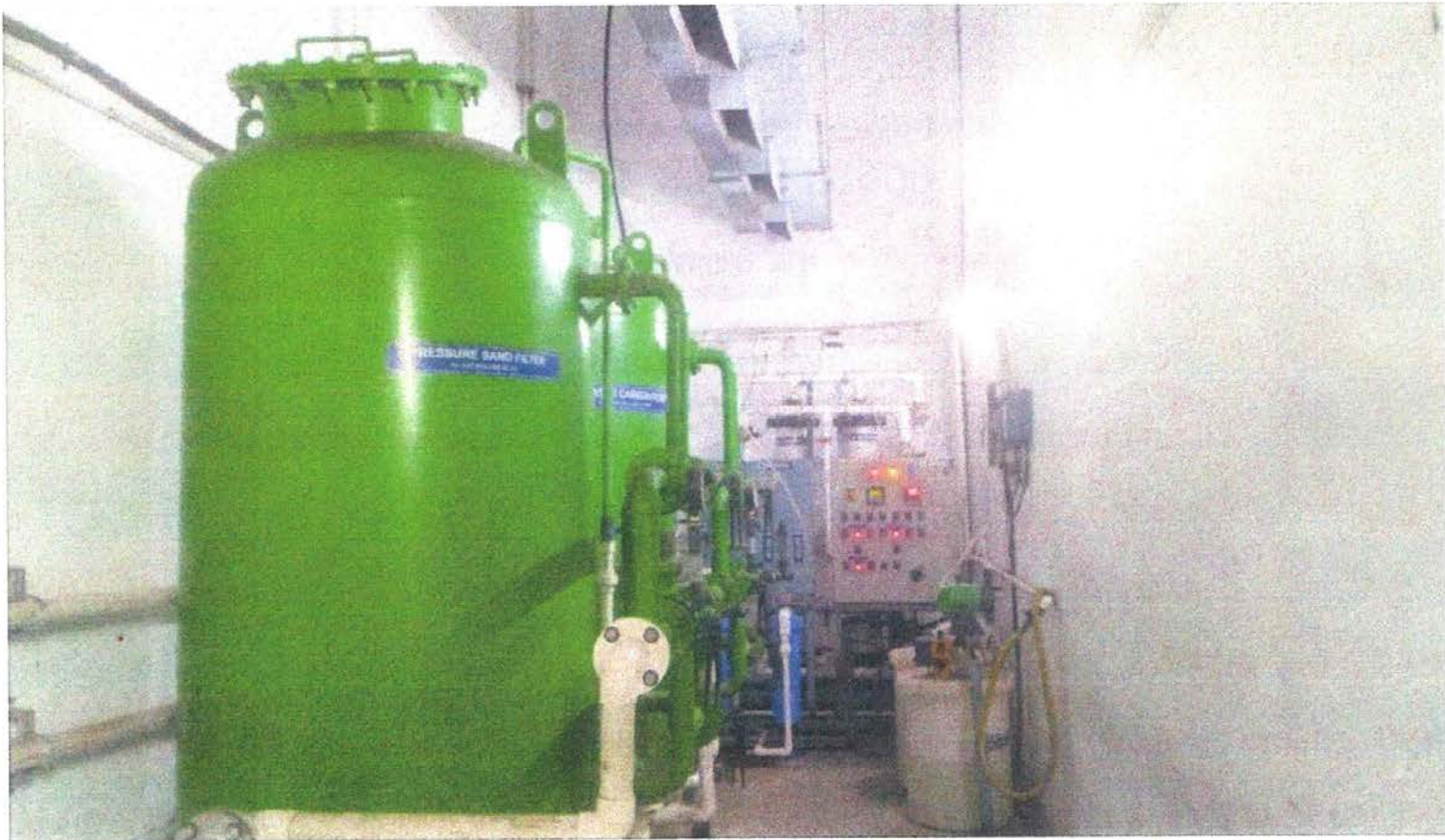
STP ROOM - PUMP
