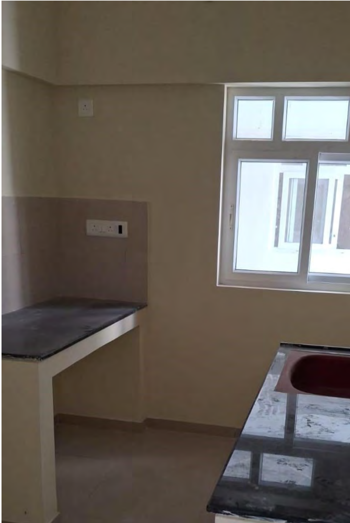
Tower B – Pic 8 – Internal Unit
