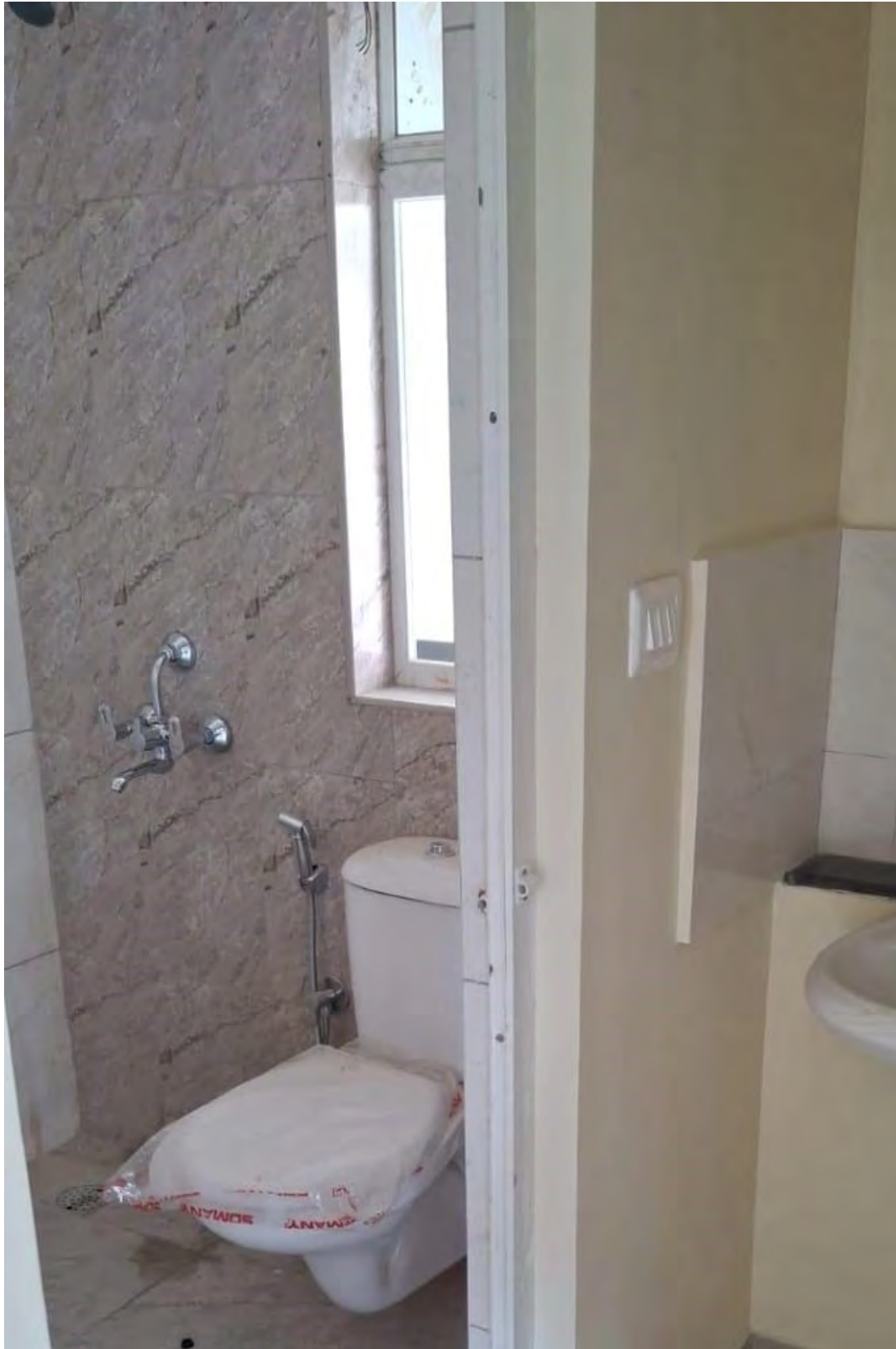
Tower B – Pic 7 – Internal Unit
