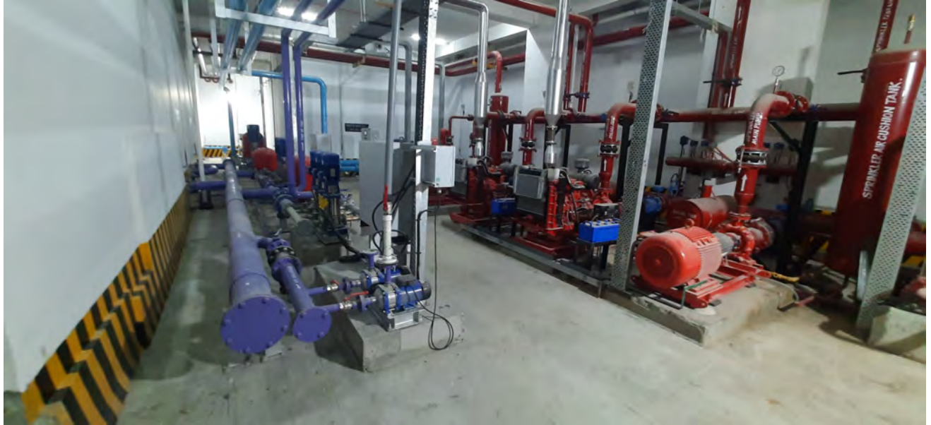
Tower B – Pic 3 – Pump Room
