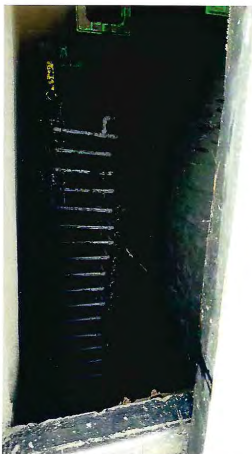
CORPORATION WATER CONNECTION
