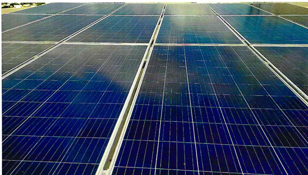
SOLAR VOLTAIC PANEL
