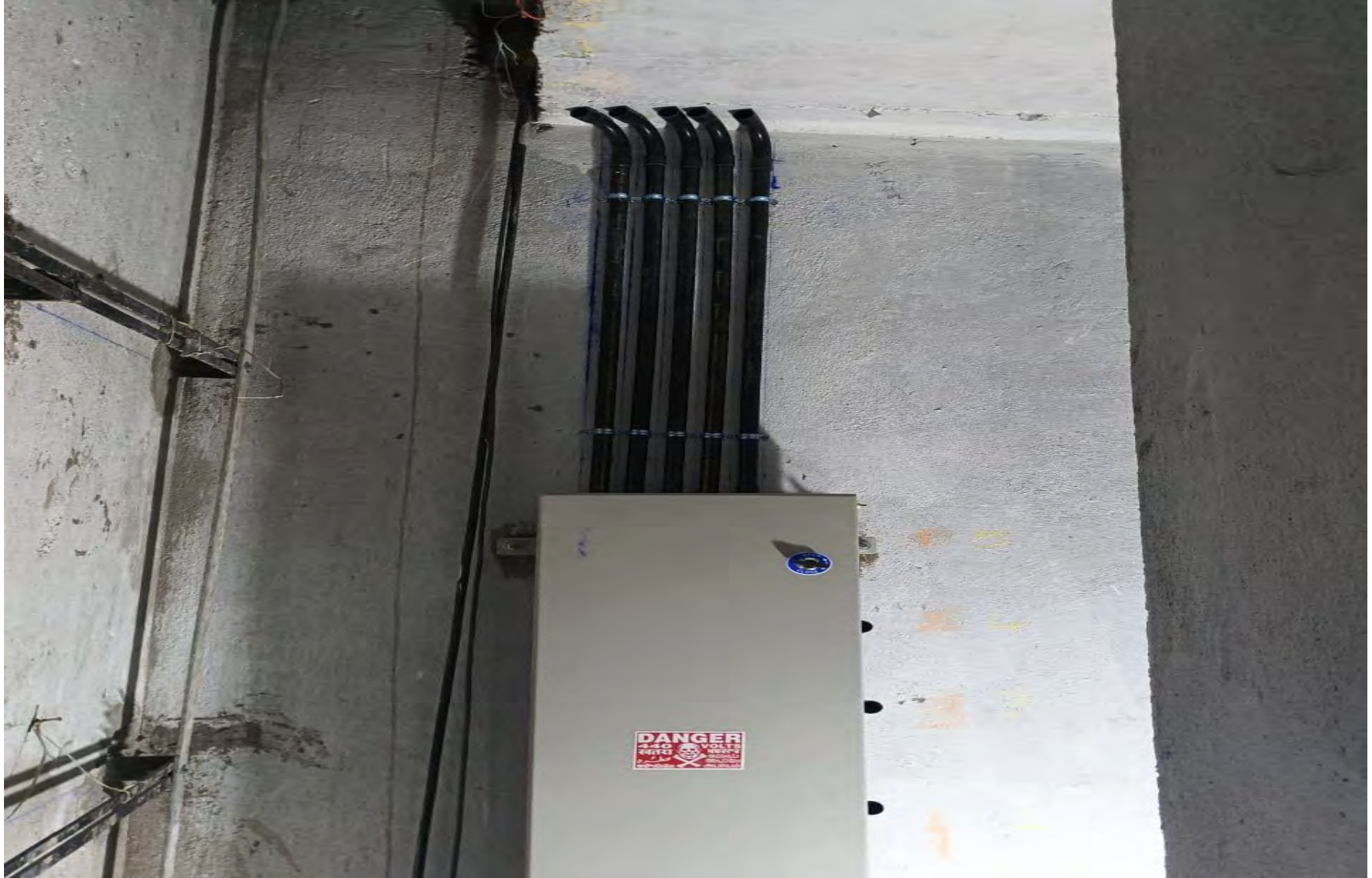
E1 A connector box in electrical shafts.
