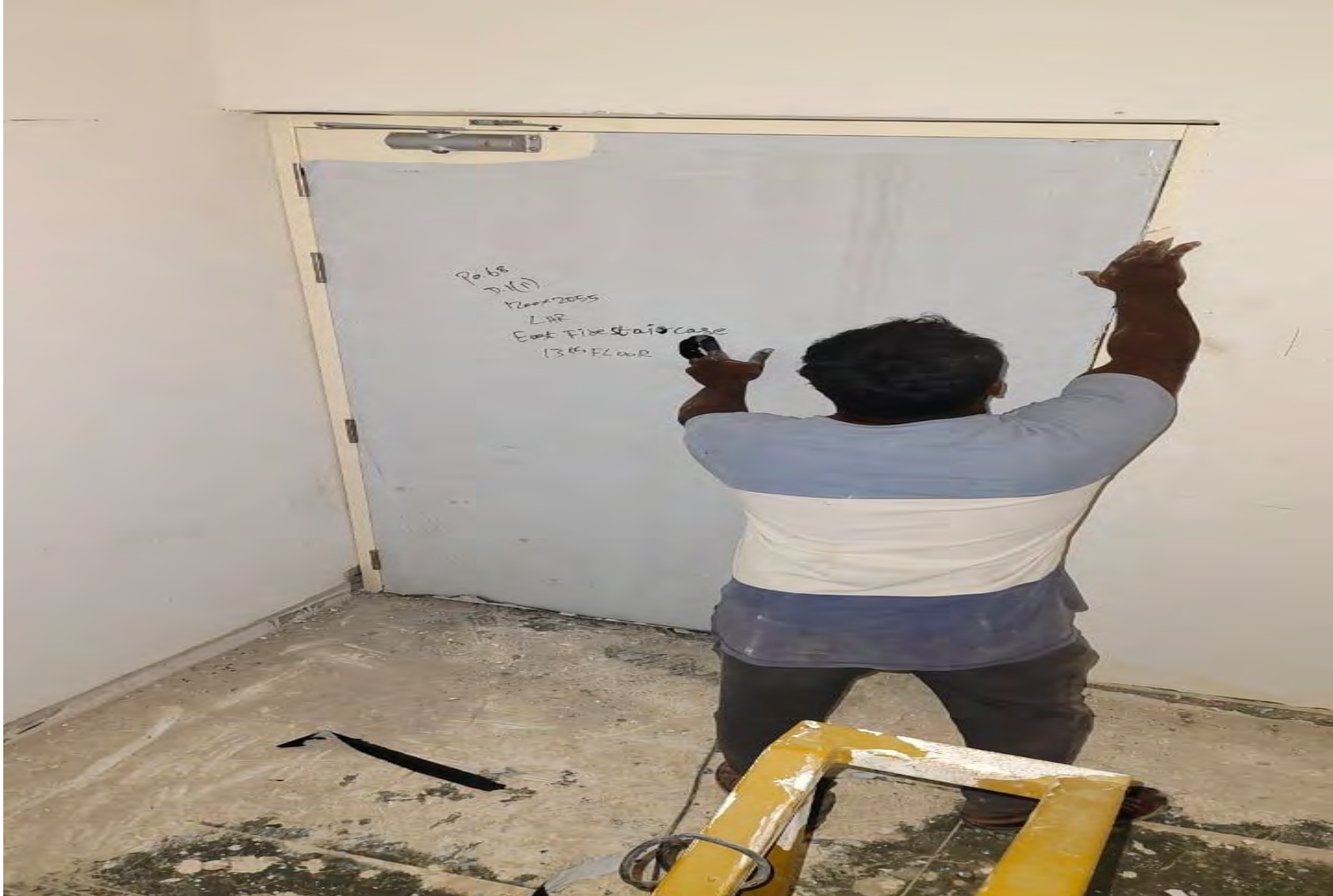
E2 1st floor- Corridor Fire exit door fixing
