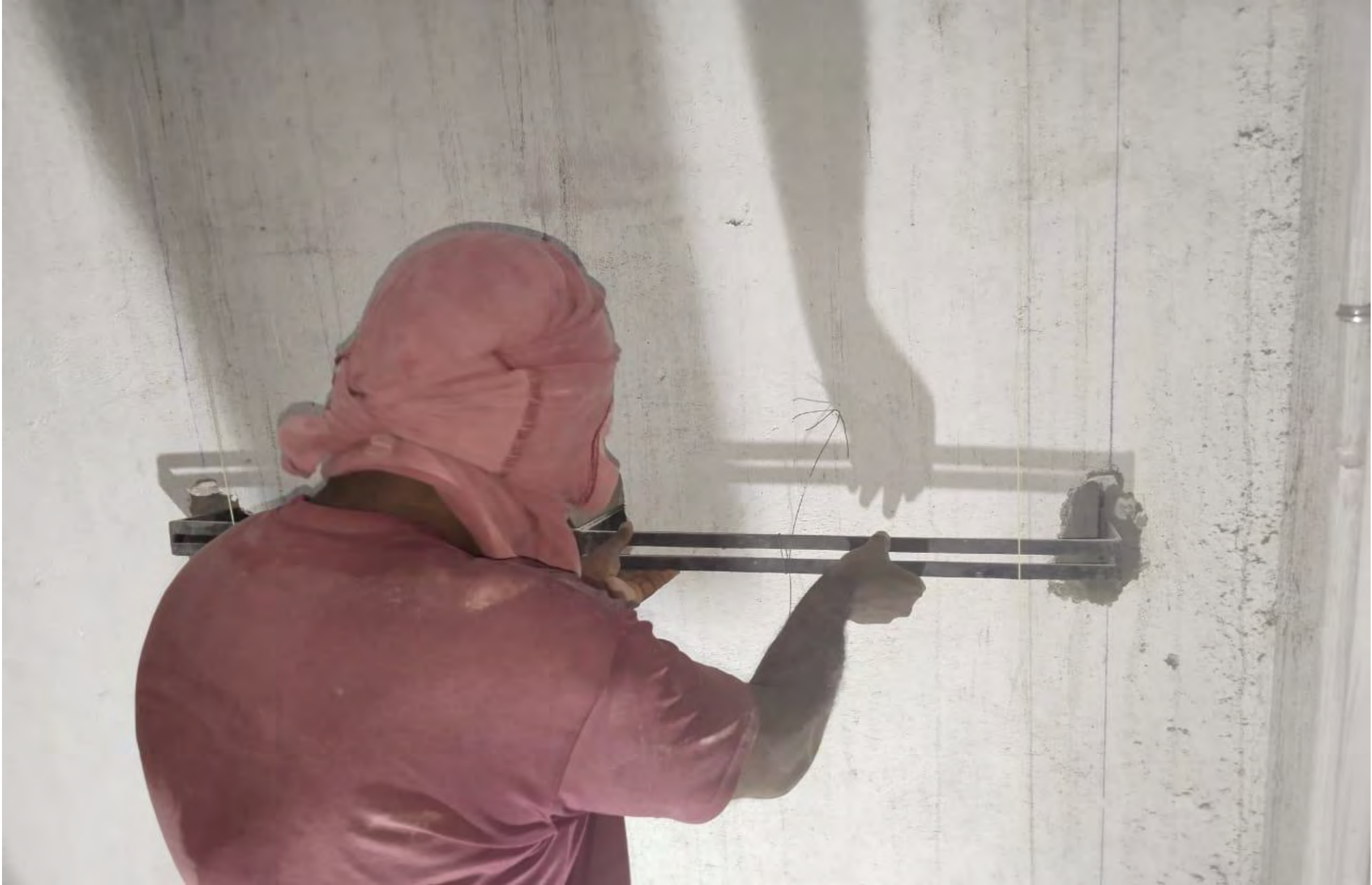
E1 B electrical shafts bracket fixing.
