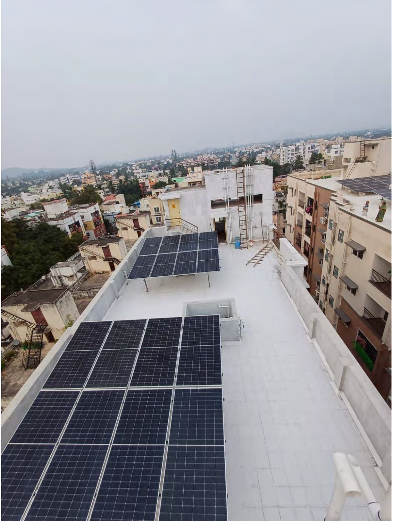
PHOTOGRAPH SHOWING SOLAR PANEL ON TERRACE FLOOR - BLOCK – A (14/01/2025)
