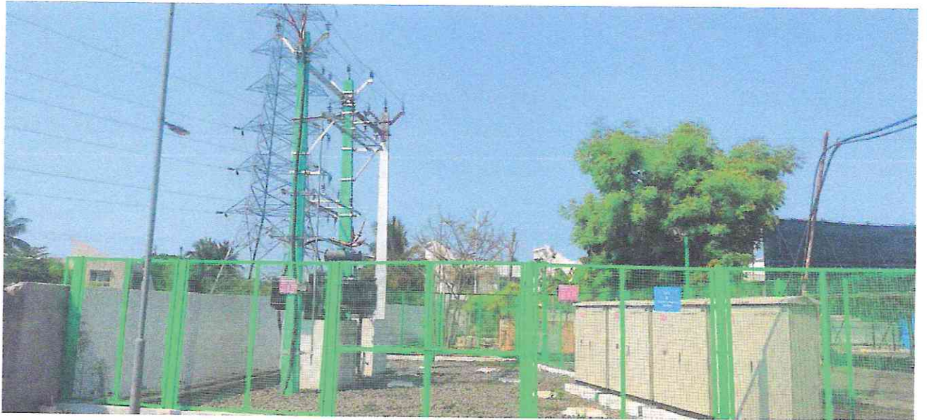
Common Services -Transformer Yard
